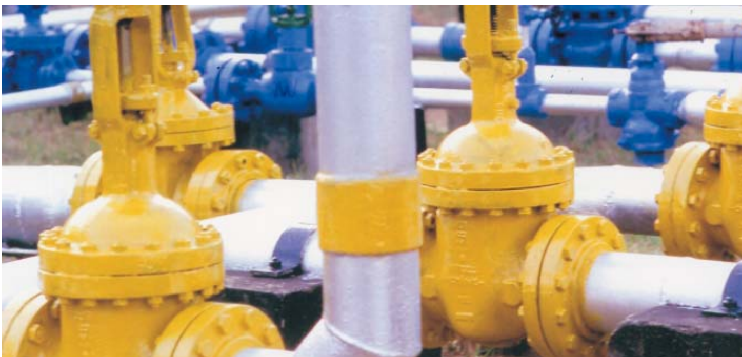
Plant piping of gas compression station of Oil India Ltd. at Duliagan
