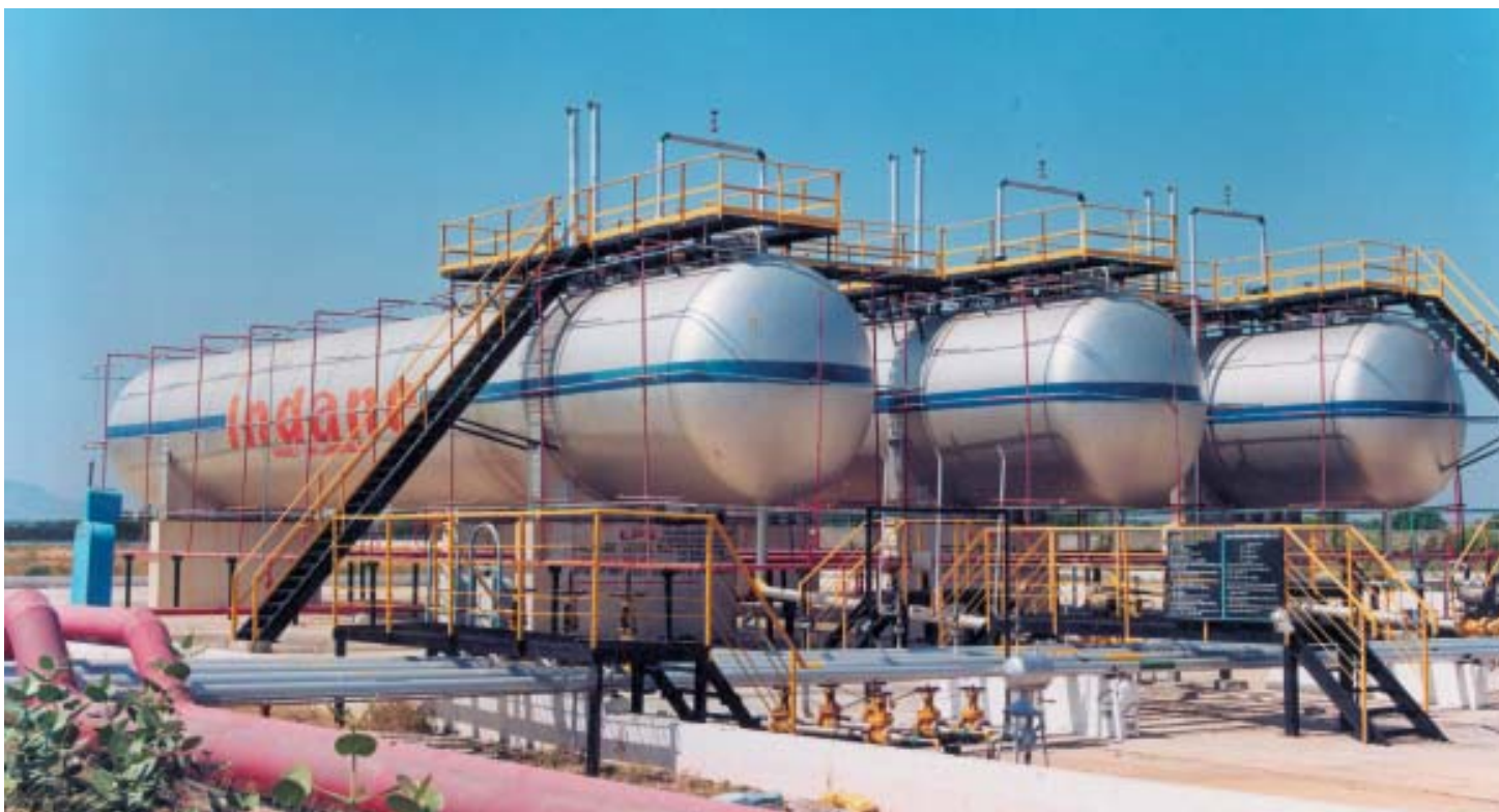
IndianOil's Indane Gas reaches 37.5 million households in the country : Pic. shows Indane Gas Bullets
