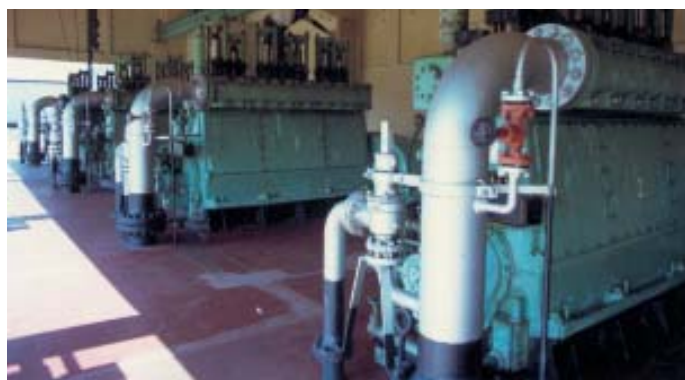
Pumping station along the Oil India's crude oil pipeline input pipeline feeding the four refineries of North-East India
