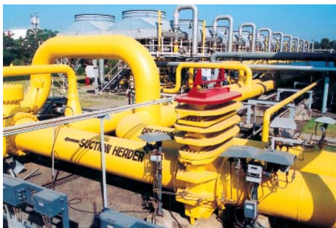
GAIL - Vijaipur Compressor Station
