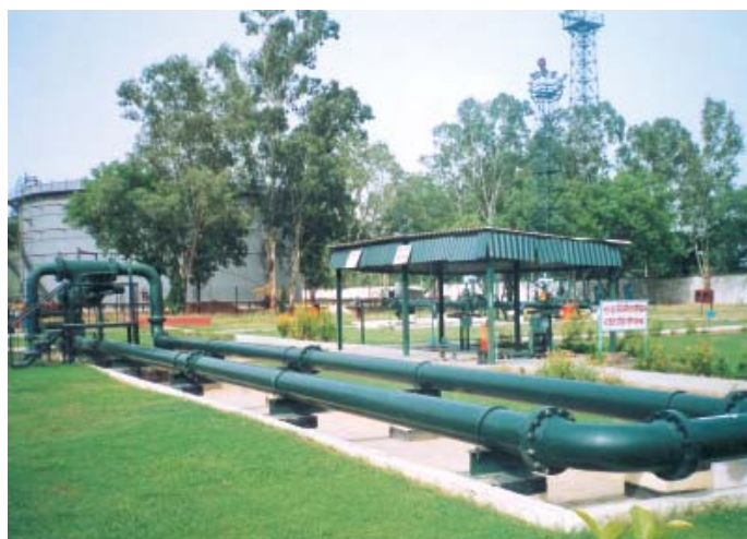
A view of IndianOil's Mathura Jalandhar Pipeline
