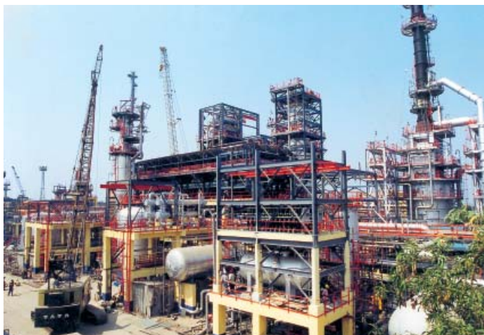
A view of BPCL - DHDS unit
