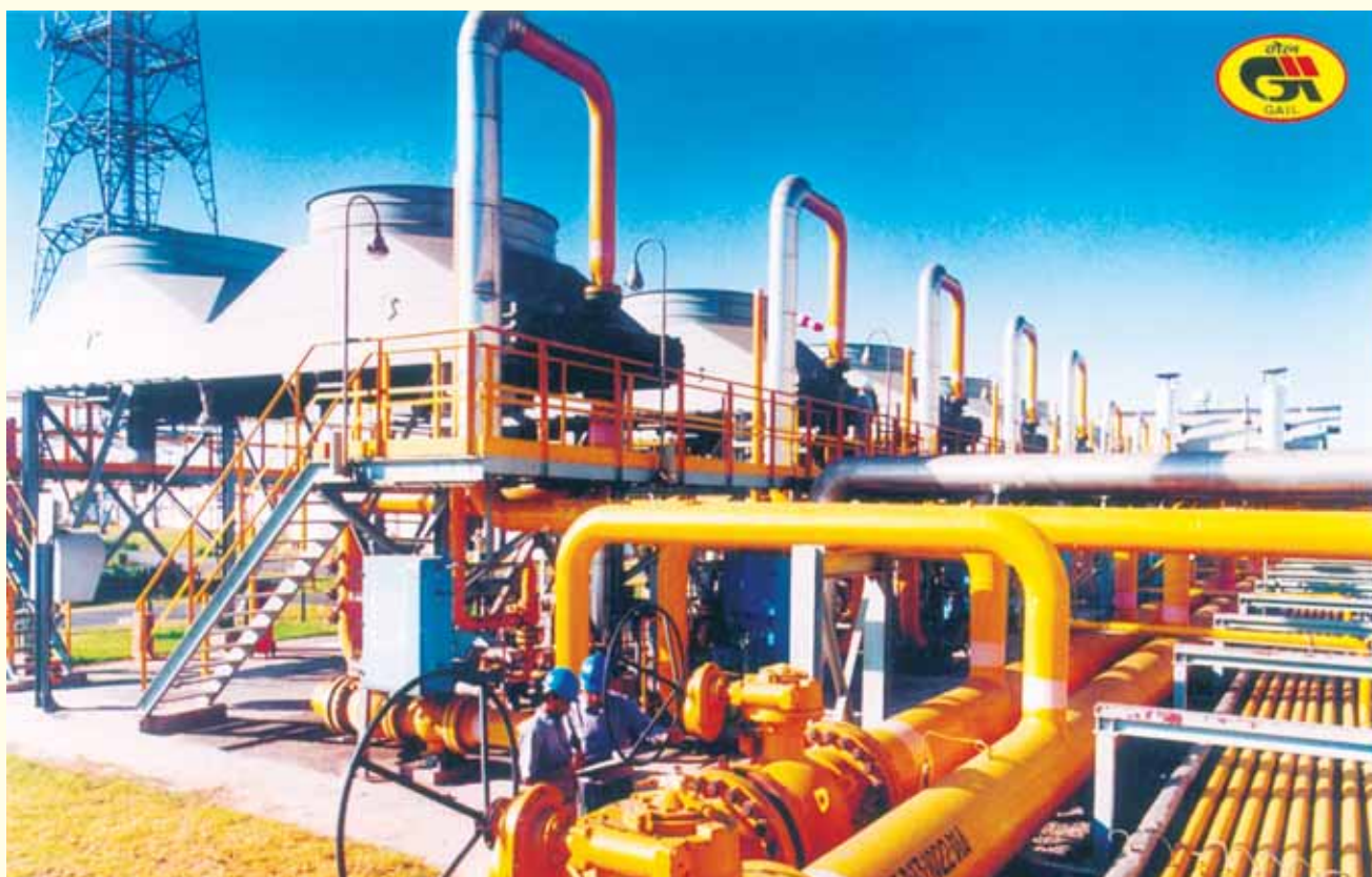
GAIL compressor station at Hazira, Gujarat
