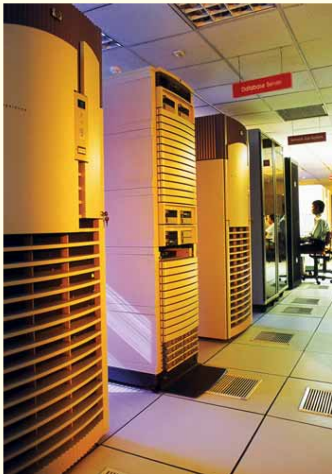
The Data Centre and Communications Hub at Gurgaon — providing online country wide connectivity for business transactions.
