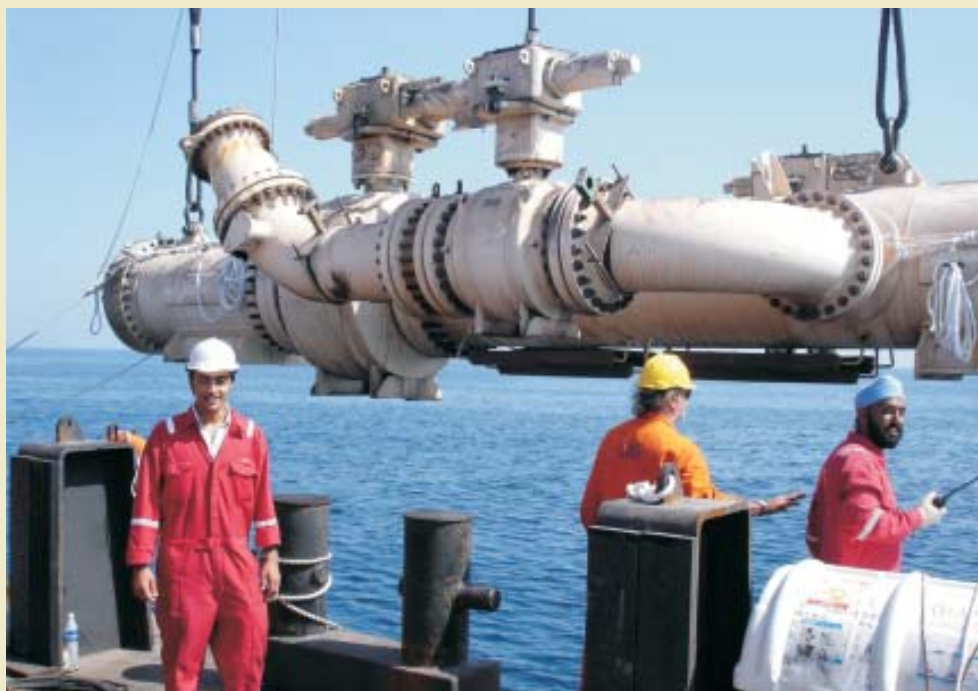
The Paradip-Haldia crude oil pipeline of IndianOil
