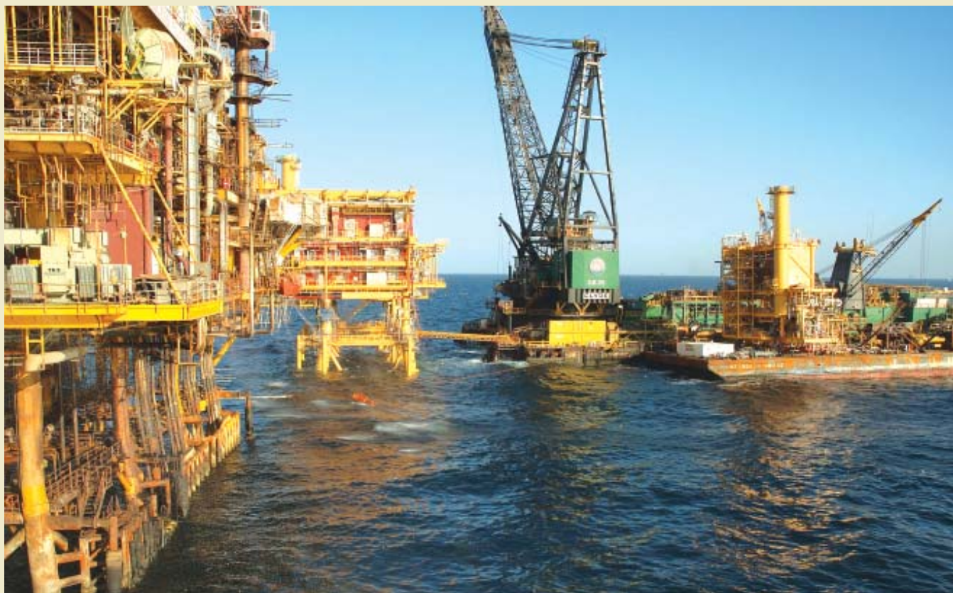
A view of an ONGC Offshore Platform in the Western Offshore
