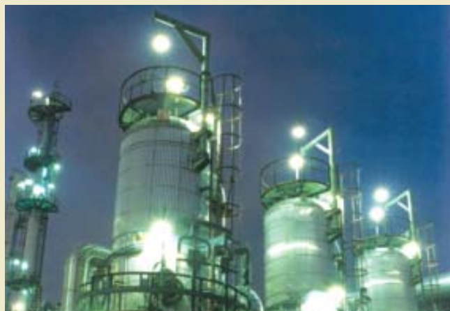
Night View of Cold Section Column of Gas Cracker Unit of GAIL at Pata, Distt Auraiya, U.P.
