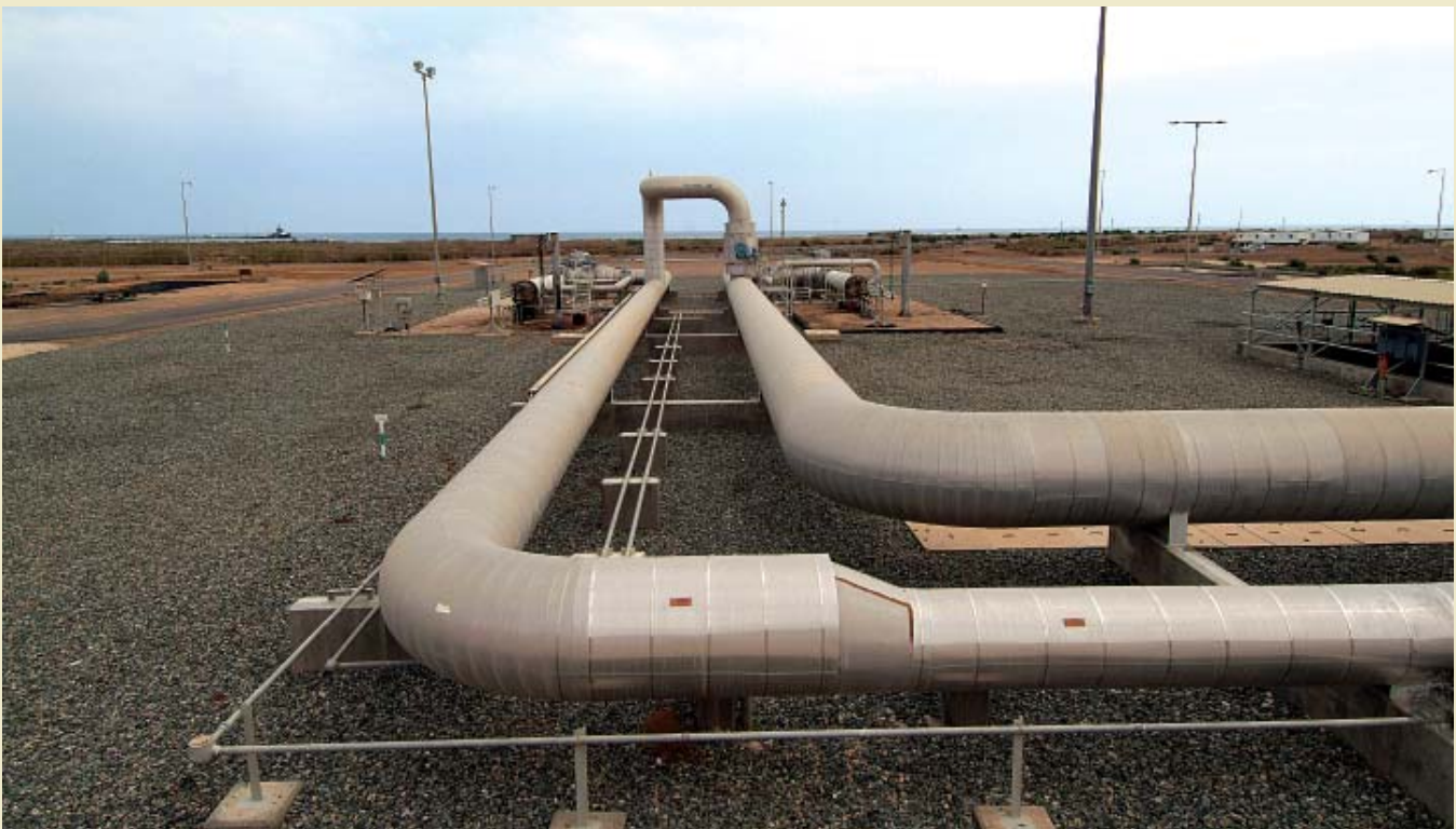
A view of Multi-product Sudan Pipeline, A joint venture of ONGC Videsh Ltd. (OVL) and Govt. of Sudan
