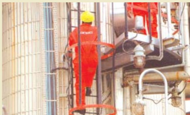
ONGCians at work at CTF, Cauvery Asset
