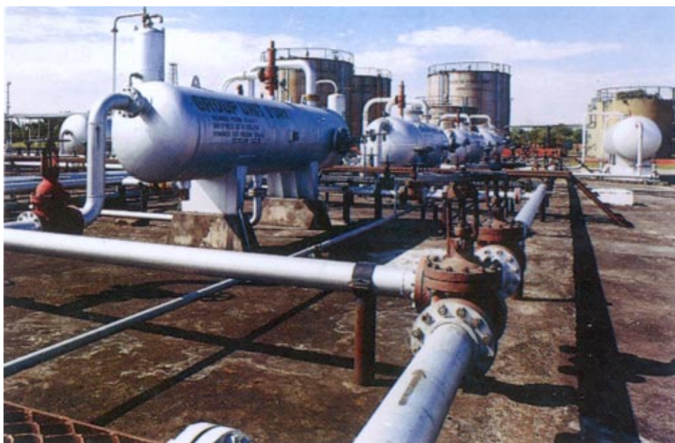
Oil Collecting Station at Duliajan of OIL
