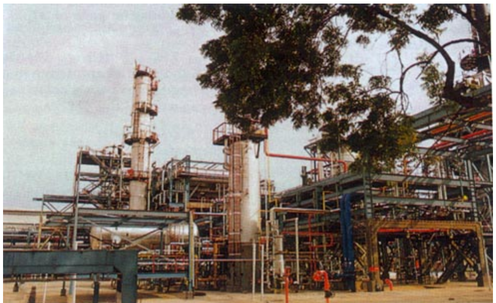
A view of the diesel hydrodesulphurisation unit commissioned at IOC's Gujarat refinery for production of extra low-sulphur diesel
