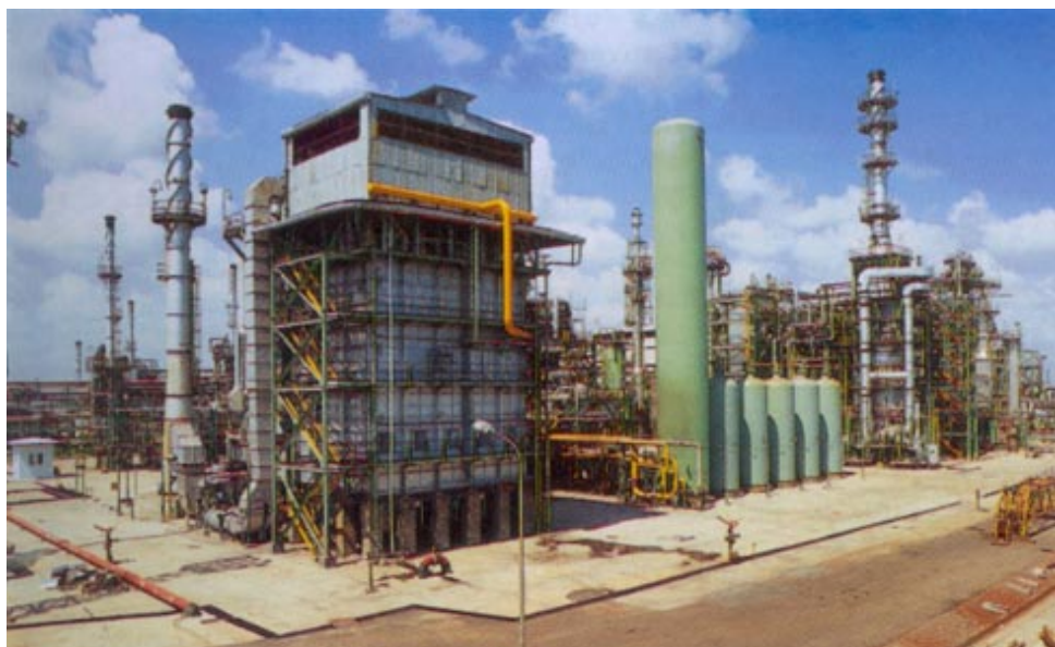
A view of reformer, PSA of Hydrogen Unit and furnace of DHDS Unit of DHDS Project of MRL
